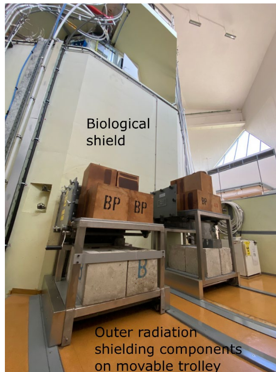
Figure 2: Photograph of the outer radiation shielding components in the reactor hall.
