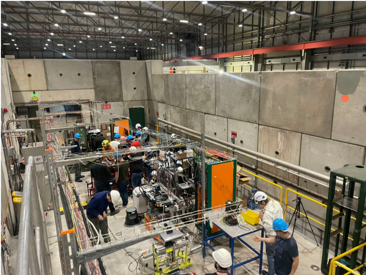
Figure 1: Installation of a user experiment in one of the experimental zones on the H8 beamline in the EHNI building.
