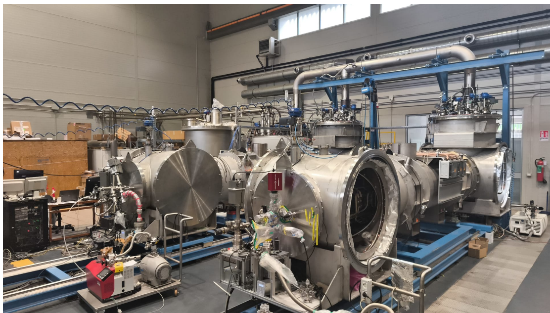
Figure 8: THOR lab and test lines, fully equipped and under commissioning (19 February 2026).
